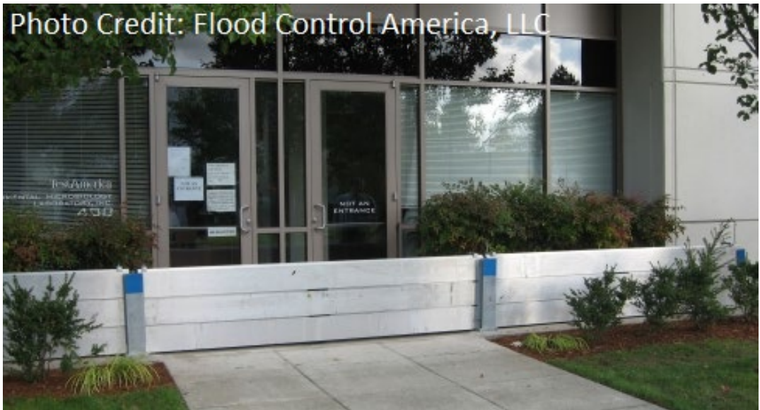
Figure 9-2. Removable Flood Barriers of an Office, Bothell, Washington
